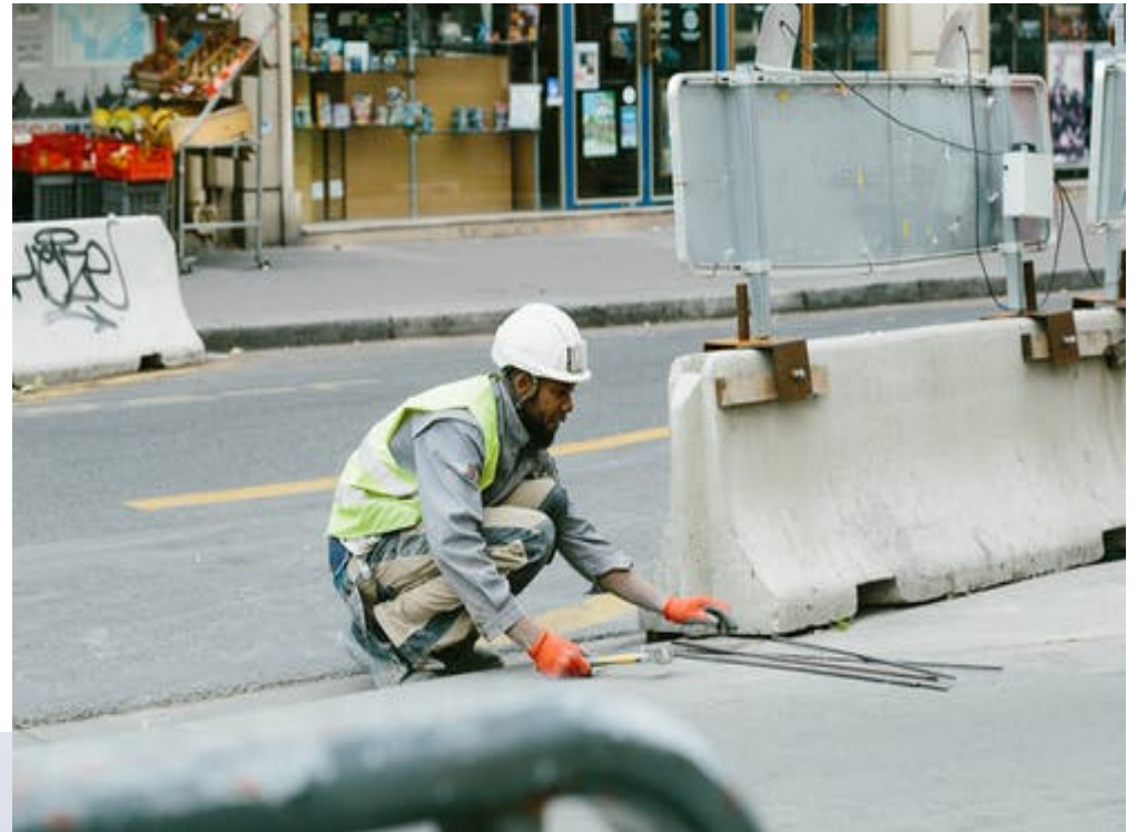
Example of use in a mobile post for road-works.
